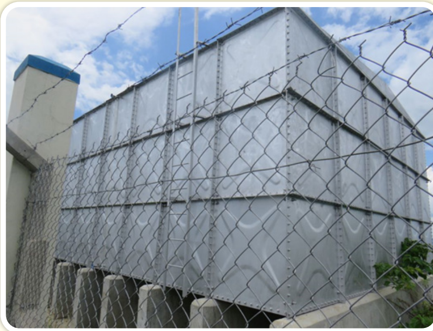
Reserve water tank
