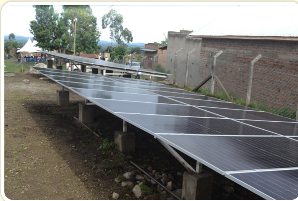
Solar panels installed at the plant, Photo by Mpamizo Evalist
